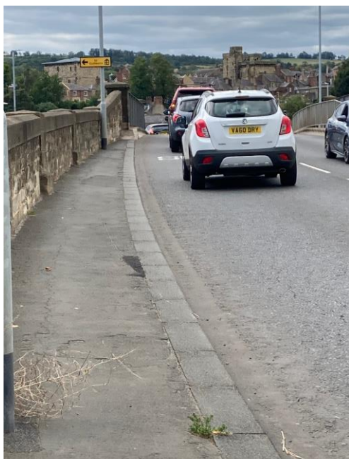
Absence of Footway Provision on Eastern side of Railway Bridge
